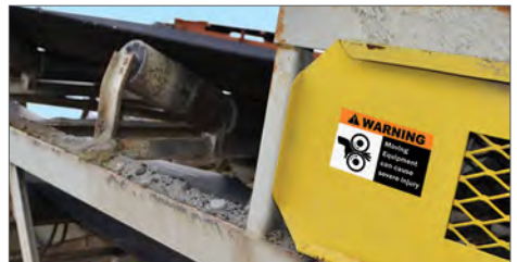
A well-placed label alerts workers to potential machine hazards.
