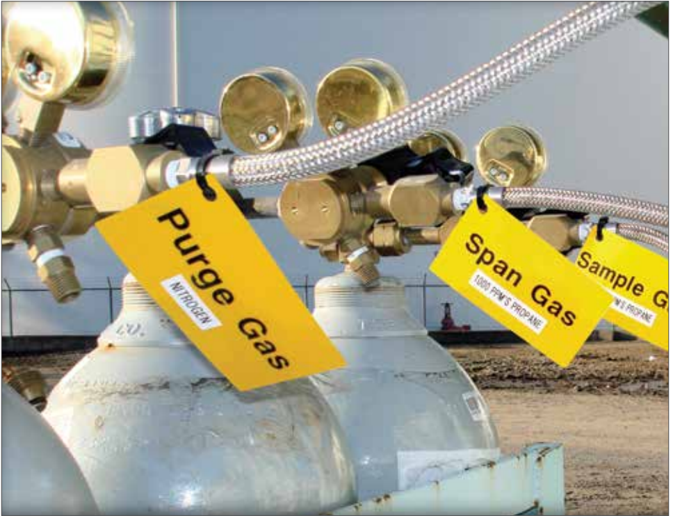
Tags may become deteriorated over time and will need to be replaced to keep up with safety codes.
