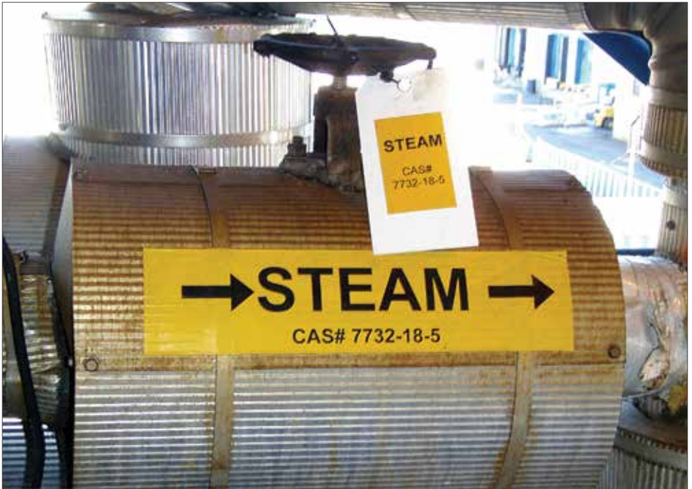
Valve tags play a vital role in safety. They can provide information for emergency responders and save lives of on-site workers.
